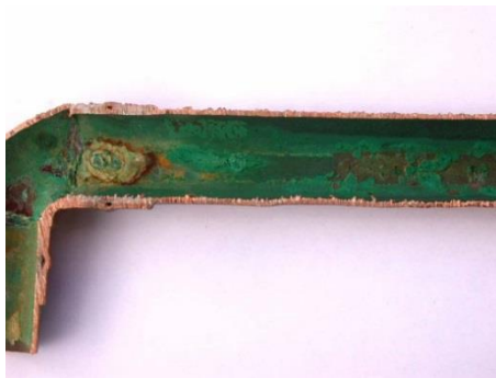
Figure 1: Crevice corrosion of copper pipe.
