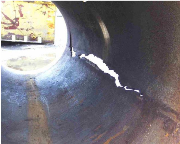
Figure 4: Stress corrosion cracking in austenitic cast iron column pipe in warm natural seawater.
