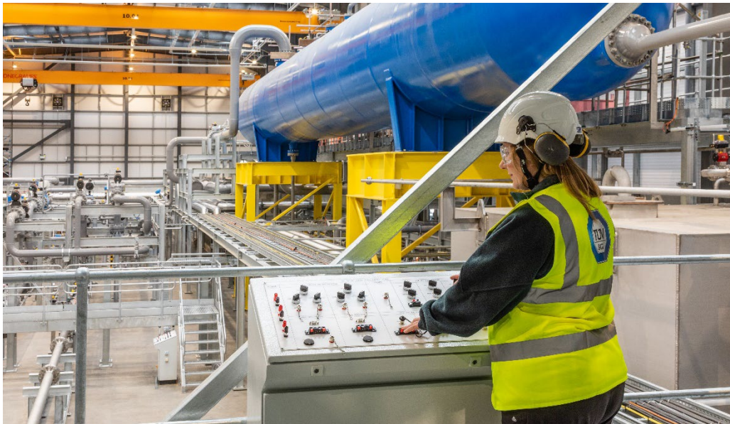
Image: Flow measurement facility
